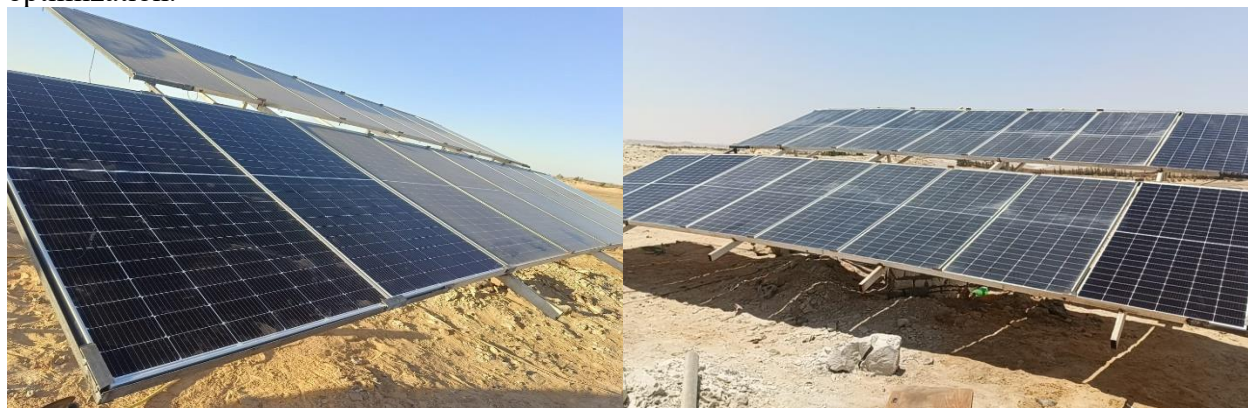
Fig. 4. 15 monocrystalline silicon PV modules, each rated at 550 W.
